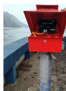
Automatic water level monitoring (vw)
