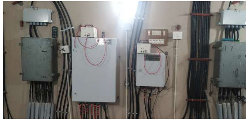
Data acquisition system
