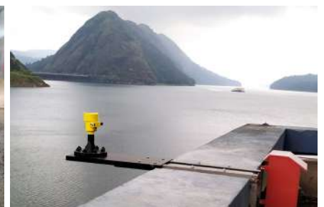
Automatic water level monitoring (radar)
