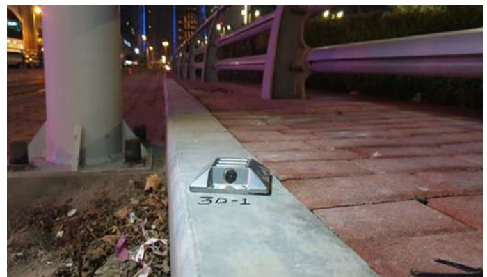
Cat-eye prism installed to monitor surface settlement along tram alignment
