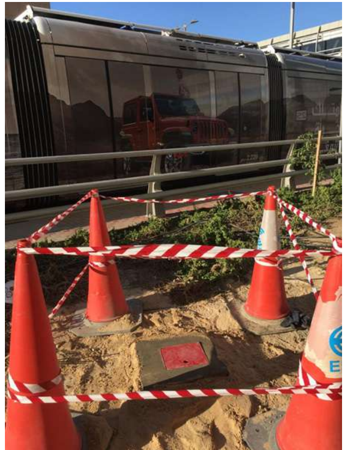
Borehole extensometer installed to monitor sub-surface settlement near tram alignment
