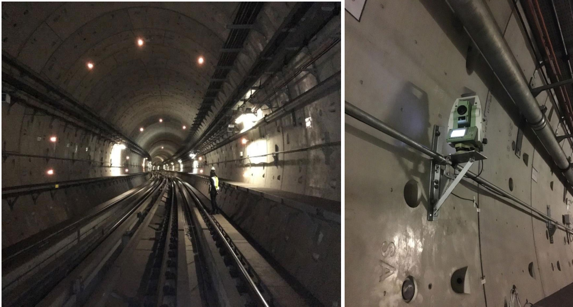
Fig. 10. Monitoring sections of a tunnel with prism targets (left) and ATS mounted on the tunnel wall
