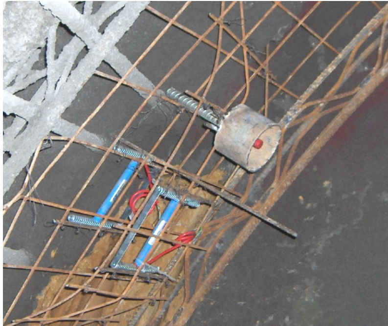
Fig. 1. A pair of shotcrete strain gages and convergence bolt of an optical target installed before shotcreting of an NATM tunnel
